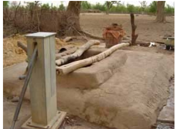
Among the projects the team completed was repairing a deep-well pump that had been broken since 1986. While in Mali, the group took the village from one working well up to a total of four sources of fresh water.
